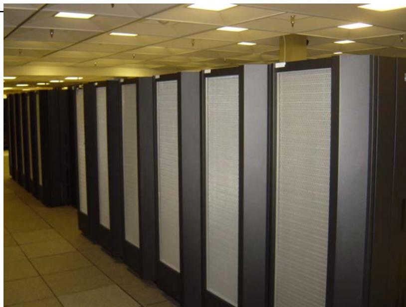
3/2011 Thermal Management Applied to Data Centers with Focus on Energy Efficiency 35
